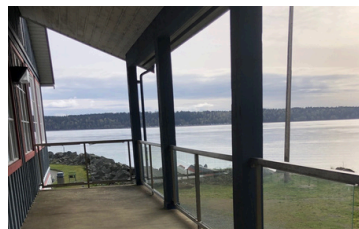
ACCESS TO DECK
